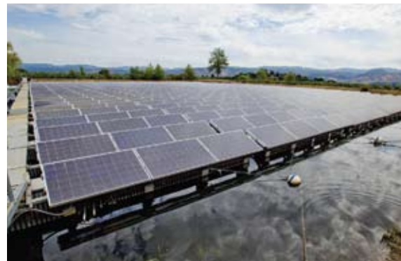
► The innovative Floatovoltaic® system at Far Niente winery
